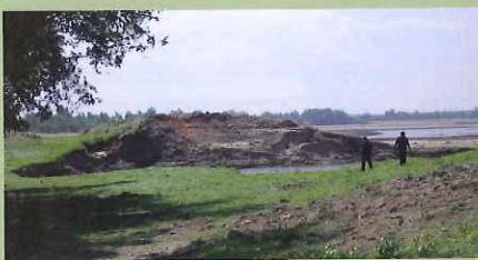
Breached levee at the upstream end of the Birds Point-New Madrid floodway.
